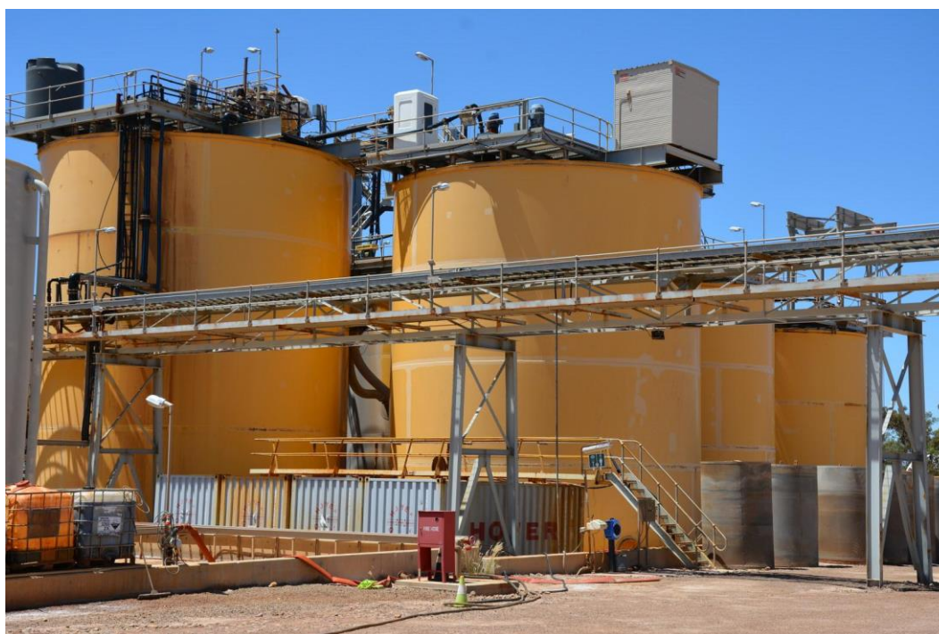
(Figure 5 - The Wonawinta Plant)
